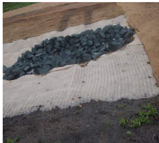
Gravel drainage outlet
