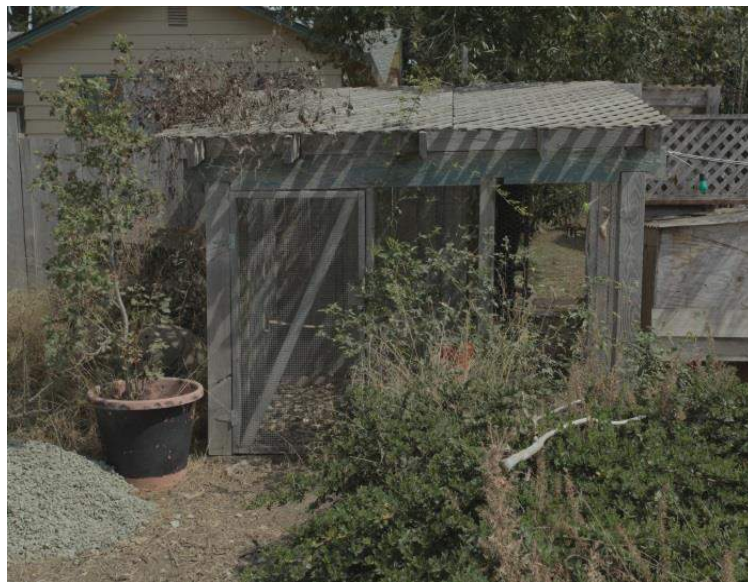
Chicken coop roof without plastic roof
