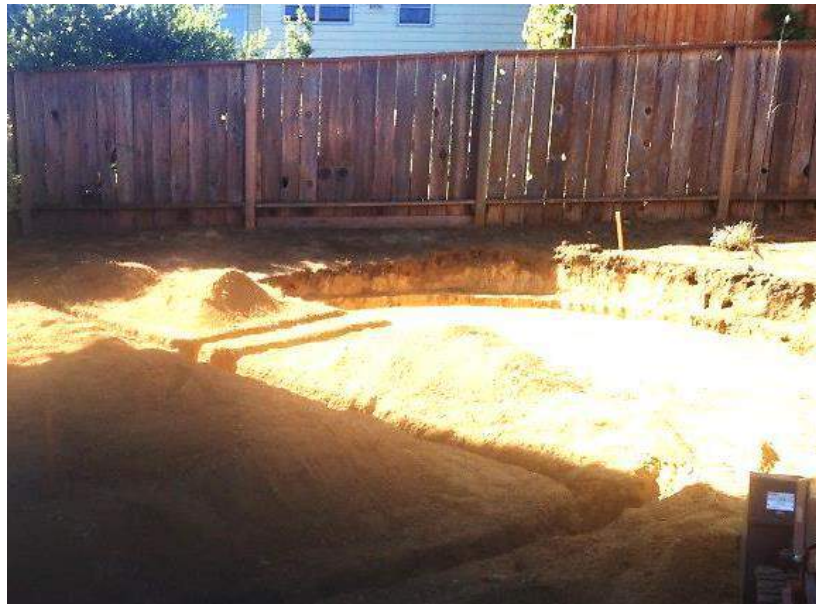
Northeast side of property showing location of rain water tanks and piping for downspouts/swale
