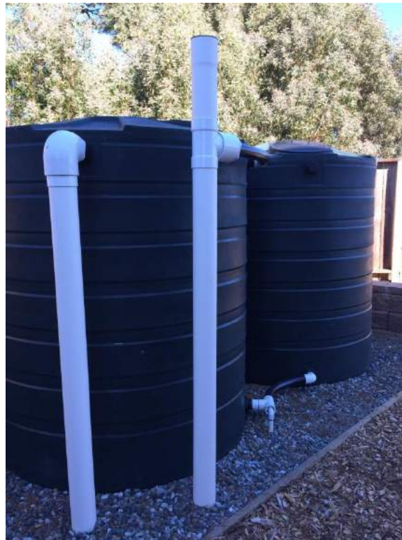
Rainwater tanks on north side of the property
