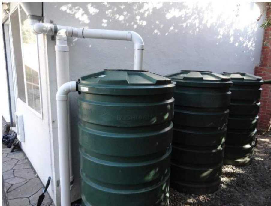
Rain water tanks with overflow to the rain garden
