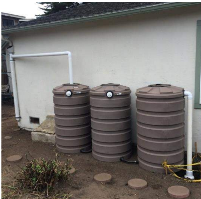
Rain water tanks on north side of property that overflow to the east rain garden
