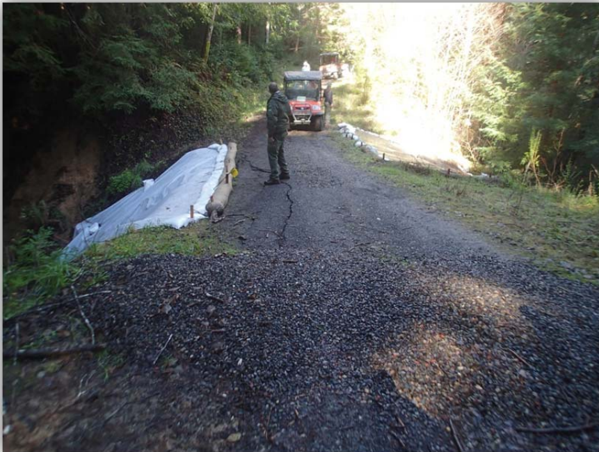
Photo 3 Photo shows cracking of road prism around upstream sinkhole. The sinkhole has been covered with plastic tarp.
