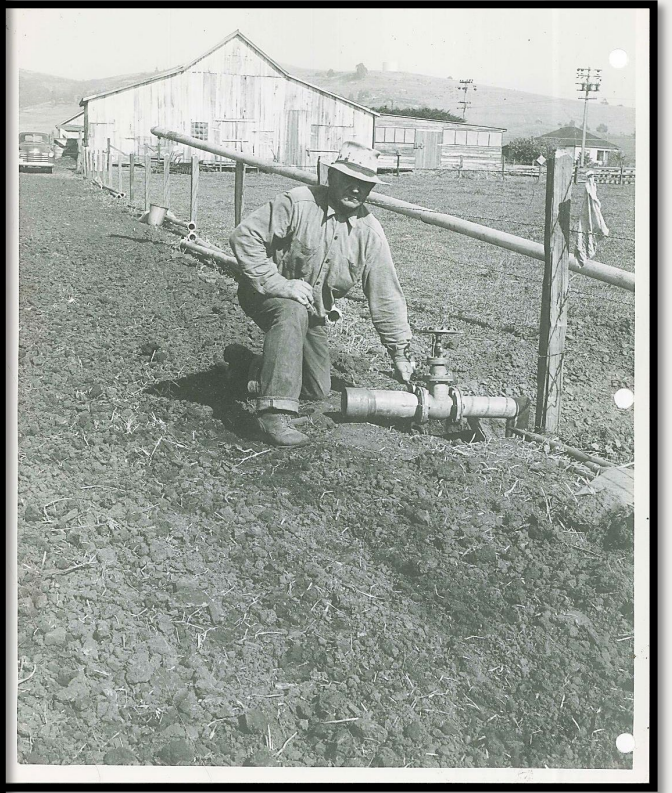
Reservoir being constructed on Farm, Half Moon Bay. Reservoir be used for stock water and irr of pasture.
